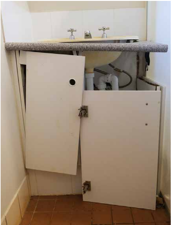
Collapsing sink basin in Remote community B
