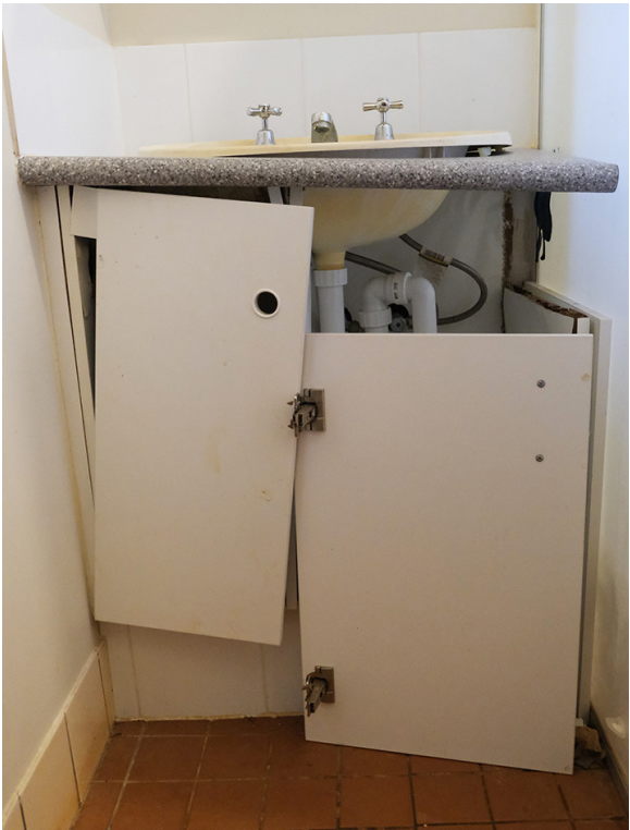
Collapsing sink basin in Remote community B
